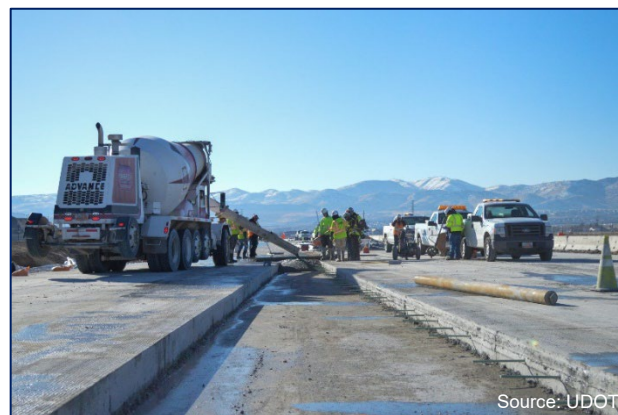
Figure 7. Highway construction in Utah. AR offers an opportunity for improved planning and ongoing management of highway infrastructure assets.
